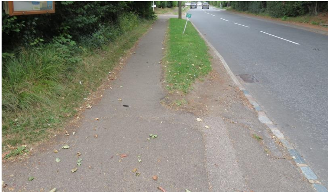
Photo 2: Looking north at the worn verge where the priority sign is to be located
